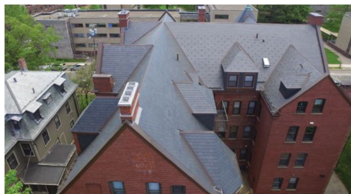
Drones can provide high resolution views of roofs and other hard-to-reach areas.
