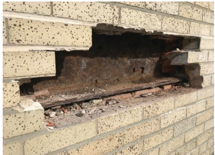
Test cuts can provide insight into the existing layers, securement methods, and material conditions.
